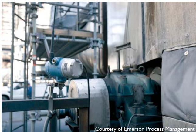
Courtesy of Emerson Process Management
