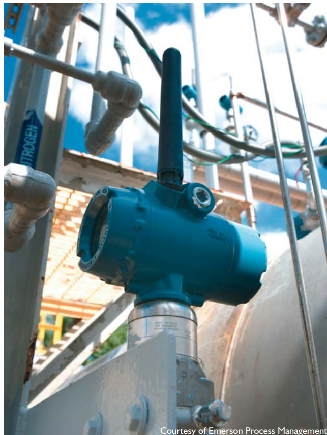
Courtesy of Emerson Process Management
