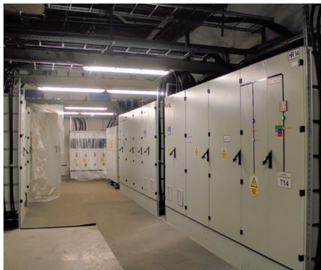
Trafostanica č.3 (T12, T13, T14)
